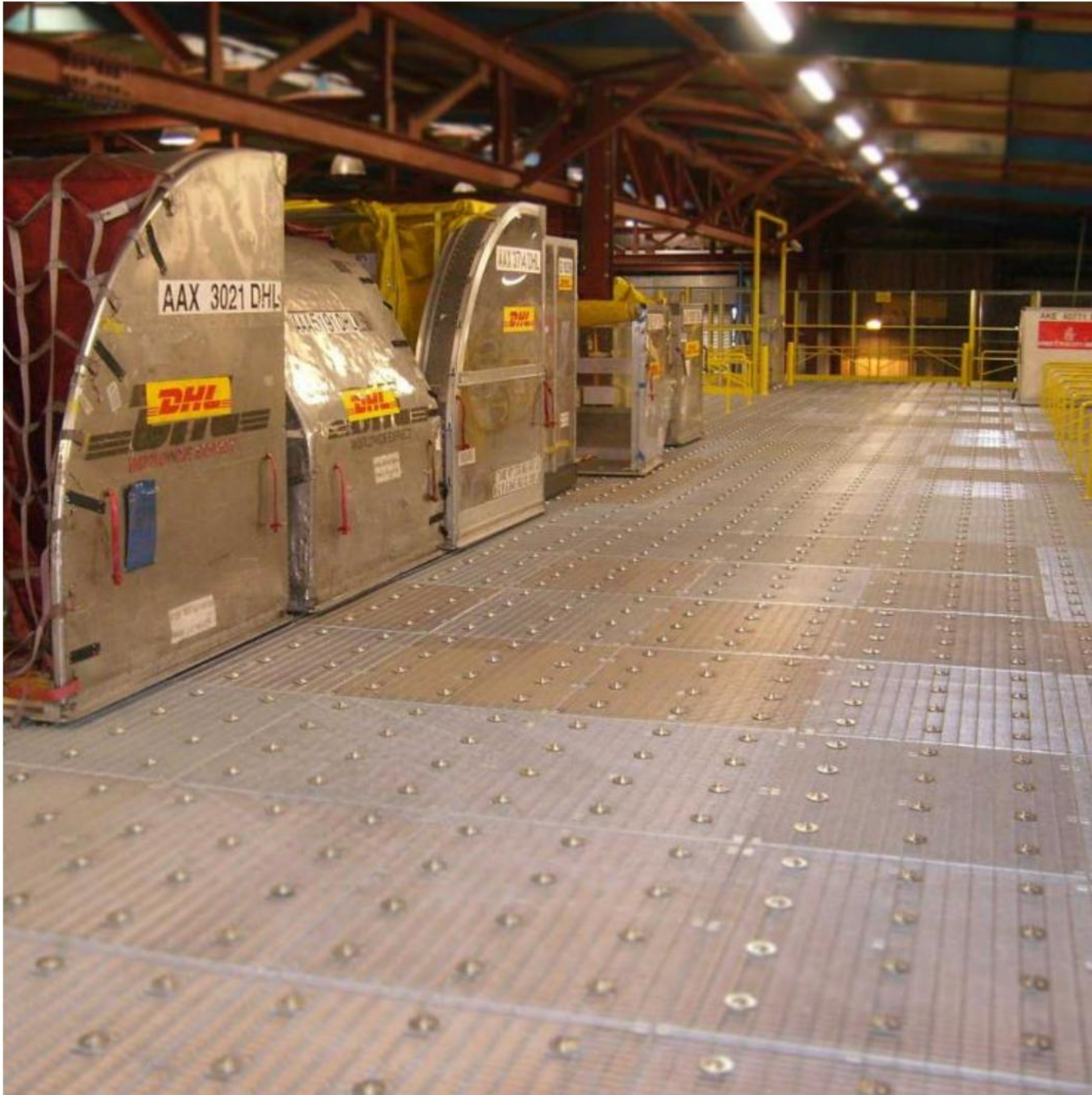
Ball Platform in DHL Heathrow Air Cargo Facility
